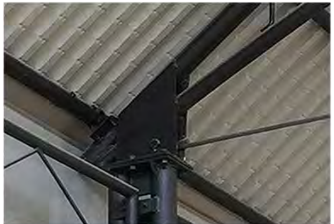
AFTER REMEDIATION WITH PANEL C
