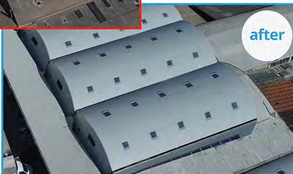
After remediation with panel C
